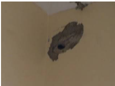
The effects of shelling on the houses in the city Alhabilayn
