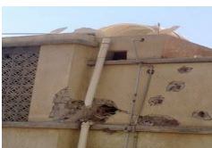
The effects of bombing on the house Atek Haythami and Abed Rabbo Haythami from the inside
