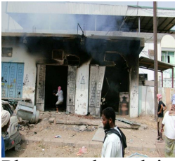
Photograph explains the gross damage happened to Jaar by bombardment of air crafts
